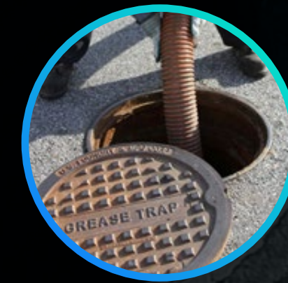
Grease Trap Manholes
